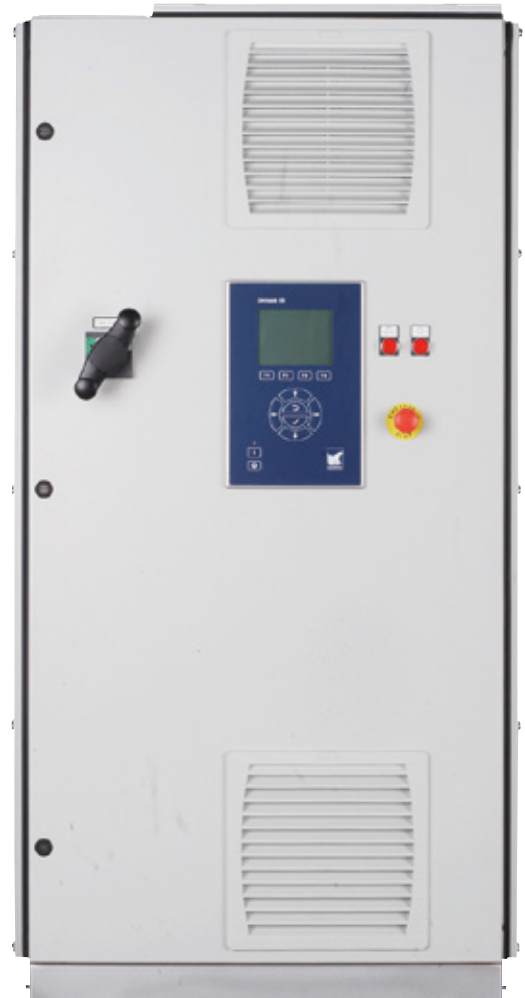
SABROE VSD panel
